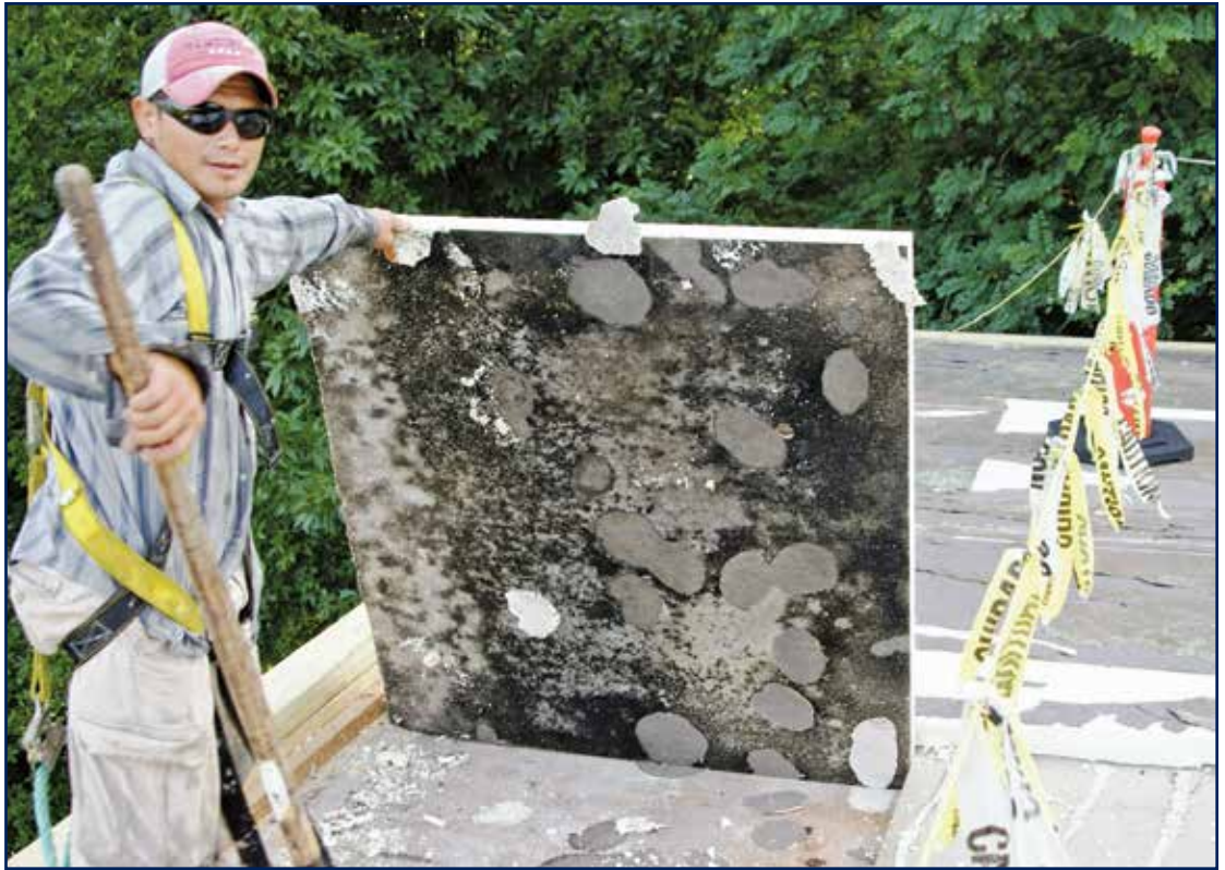
Figure 12 – Regardless of what the static dew point analysis may suggest, a vapor barrier should be reconsidered in new construction or where an existing deck has been wet for extended periods.
