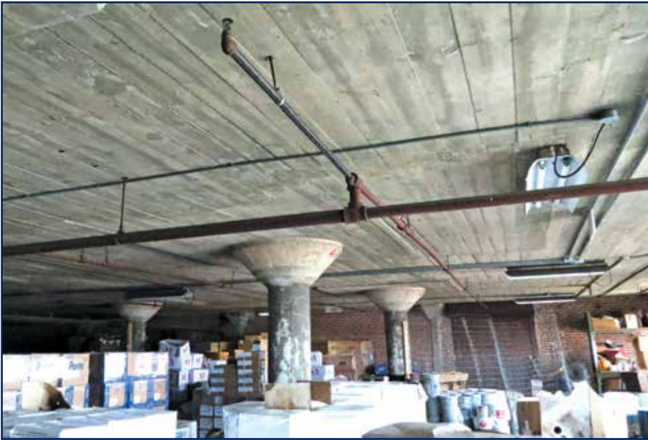
Figure 4 – Here the concrete is cast monolithically with the column capitals. This arrangement was common in multistory buildings in decades past.
