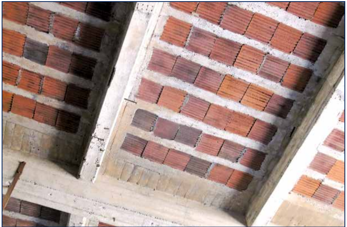
Figure 10 – Concrete roof decks may be poured over structural clay tile (also called “book tile”) situated between concrete beams and columns.
