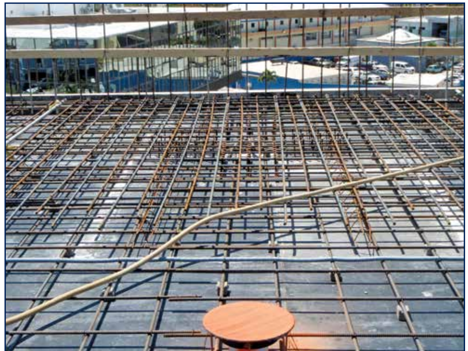
Figure 1 – The network of internal reinforcing steel for a project that will soon receive the concrete pour. Note the temporary forms that will later be stripped from below.
