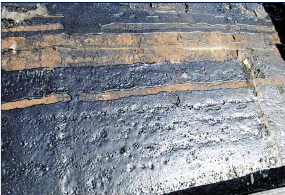
Figure 11 – Hot bitumen was—and continues to be—a plausible adhesive for insulation on concrete decks. This image, however, depicts poor (virtually nonexistent) adhesion of a roof that was installed over an old vapor retarder surface following tear-off.
