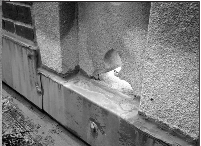
Photo 11 - Area of stone infill on roof side of parapet wall required to accommodate revised height of finished gallery roof.
