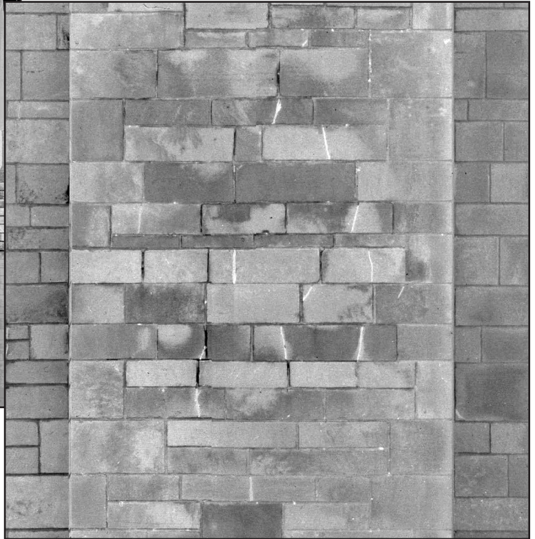
Photo 7 – Enlarged area of localized distress below tower balcony roof with failed drain leader.
