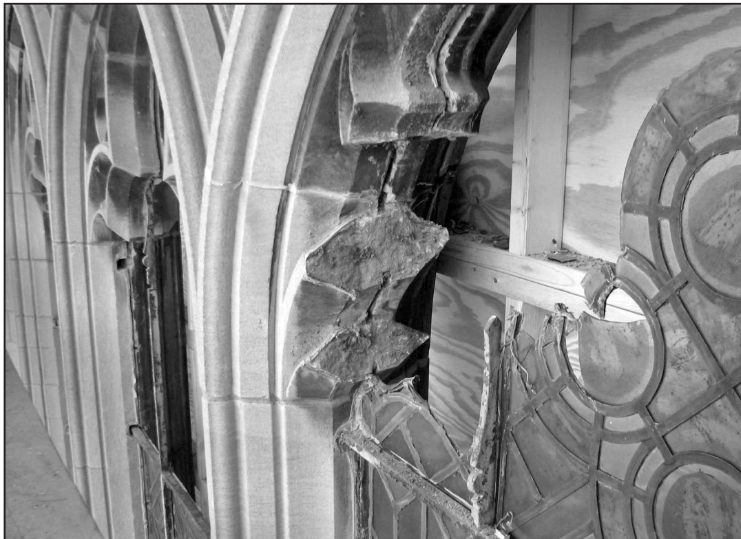
Photo 12 – At some locations, the stained glass and exterior support framing provided supplemental support to damaged stone tracery.
