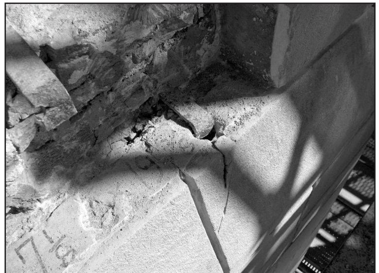
Photo 8 – Typical stone distress resulting from corroded steel strap and/or the open cell (receiver) in the stone subjected to freeze/thaw damages.
