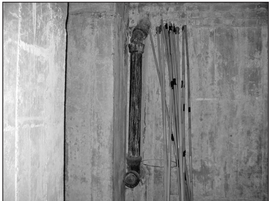
Figure 1, Condition C – Typical drain leader exiting the confines of the buttress as presented in the basement.
