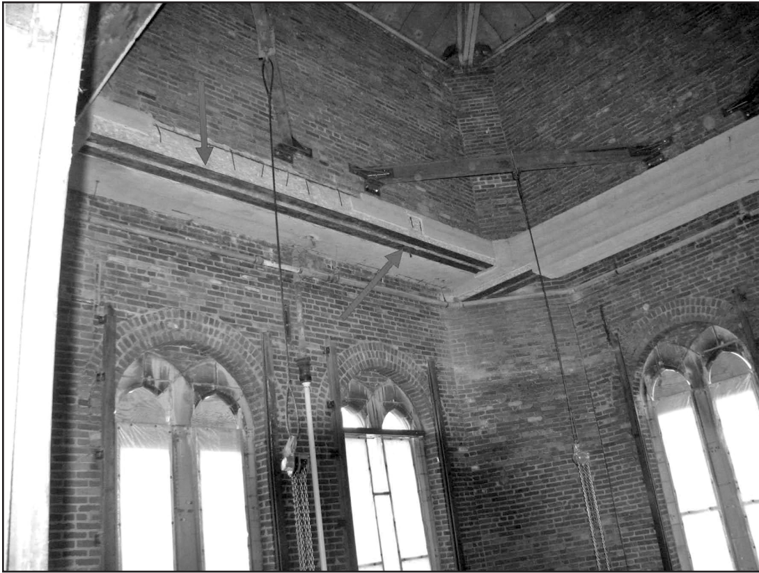
Photo 15 – Loss of concrete cover (fireproofing) at upper tower limits resulting in recurring water entry.
