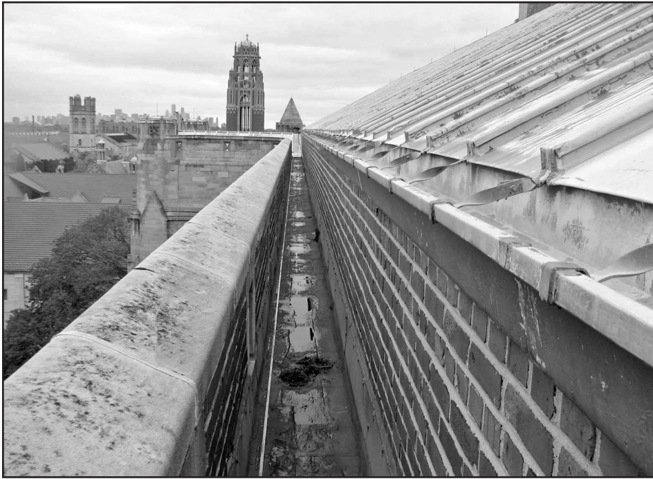
Photo 9 - Typical integral gallery at the east and west sides of the nave.
