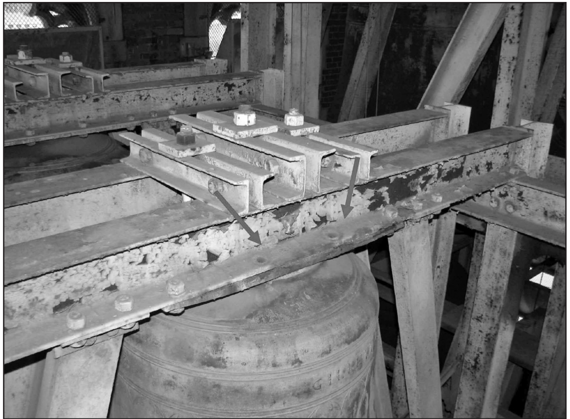
Photo 19 - Wind-driven rains entering the tower interior, resulting in heavy corrosion of steel plates and failure of bolted connections.
