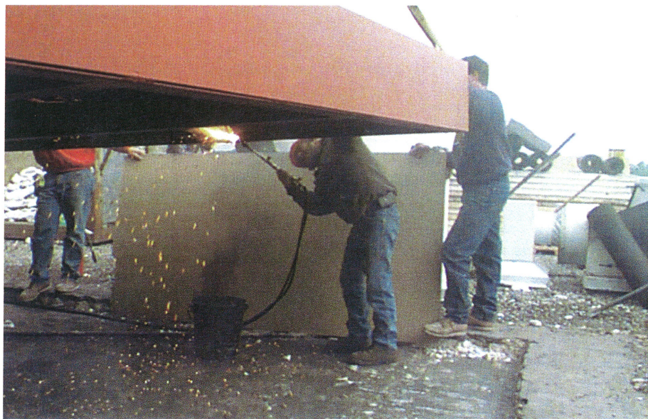
Small fire contained in bucket.
