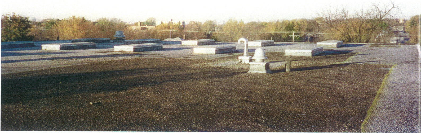
Overall of a fairly large anomaly in a built-up roof assembly.
